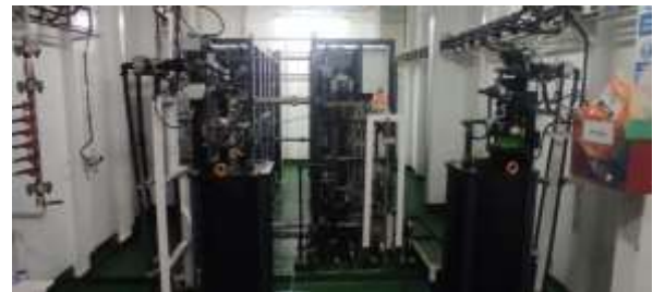
Gambar 3. 4 Water treatment unit
